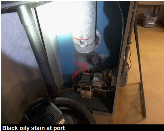
Black oily stain at port
